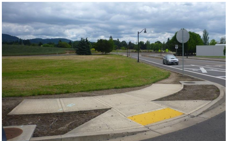
ADA Compliant Curb Ramp with No Connections
